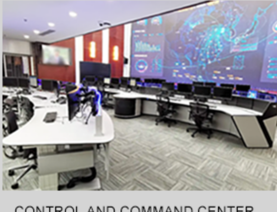
CONTROL AND COMMAND CENTER
