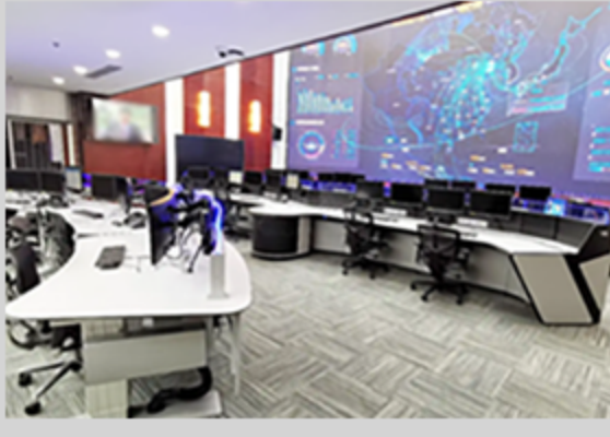
CONTROL AND COMMAND CENTER
